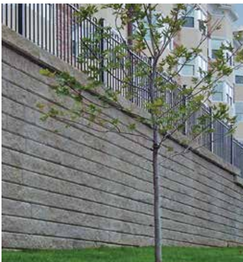
Fence incorporated directly above wall
